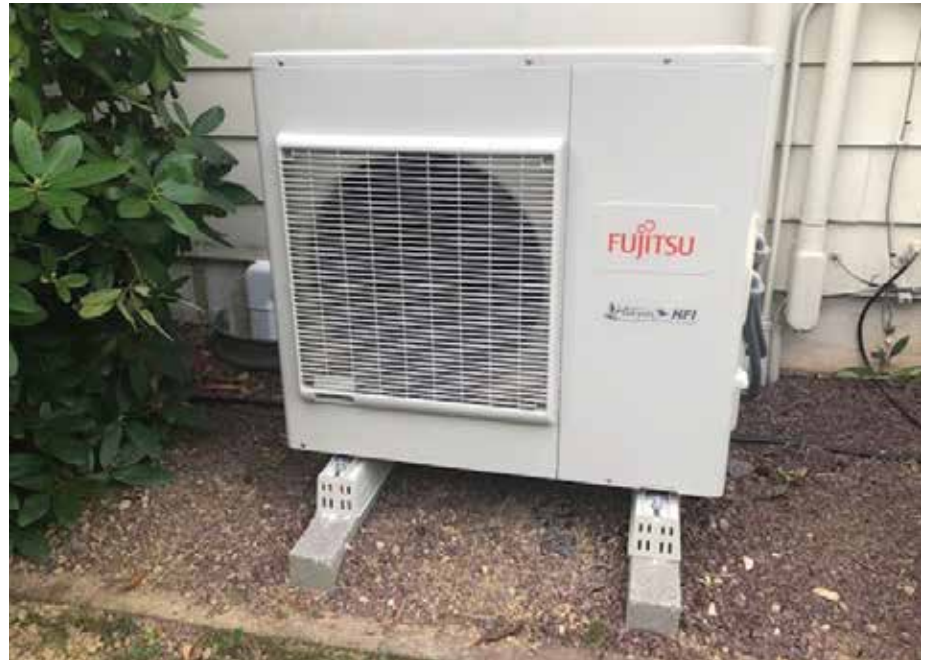
ELIGIBLE FOR A REBATE: Mini-split systems have become extremely popular with consumers looking to save money. Bedford REC members who buy and install these and other alternative heating and cooling systems are eligible for rebates.
