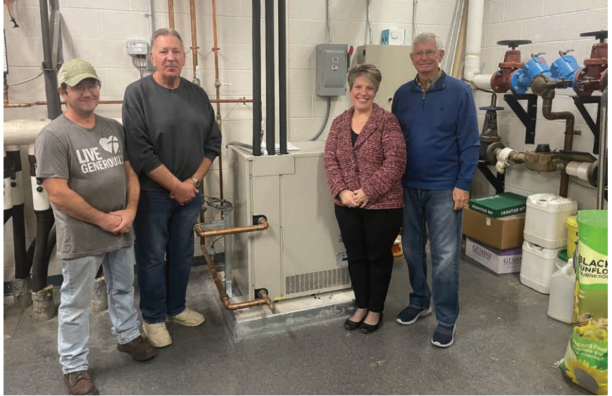
START UP: From left, Mike Freeman, Rick Cessna, Leah Pepple and Dan Koontz stand next to a newly installed Variable Refrigerant Flow Unit, one of many energy-related upgrades made recently at Allegany College of Maryland's Bedford County Campus.
