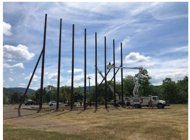
SETTING THE STAGE: A Bedford REC crew sets poles for what would eventually become the Silver-Lining Drive-In movie screen at the fairgrounds in Bedford.
